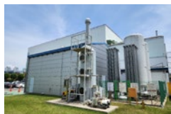
Air Pollution Prevention Facilities - Dust scrubbers
