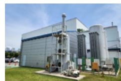
Air Pollution Prevention Facilities - Dust scrubbers
