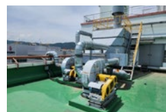
Air Pollution Prevention Facilities - Activated carbon adsorption facility
